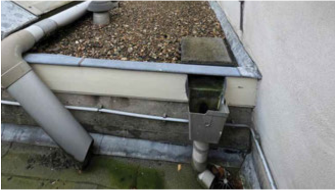
5 Down pipe system | urgent improvement needed
