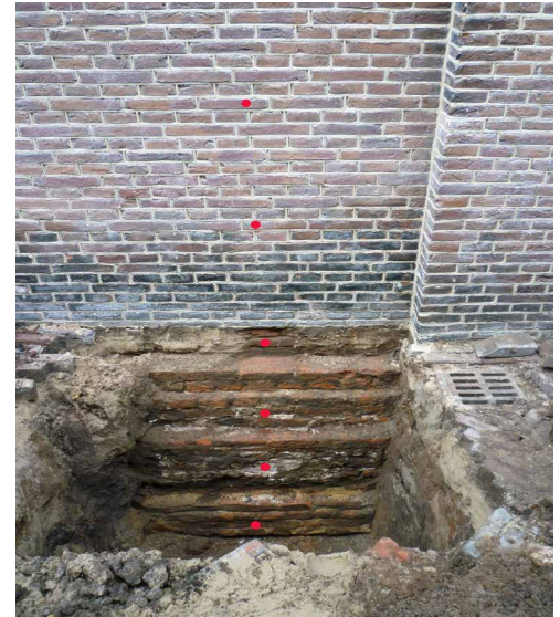
FIG. 3.13 Excavation of the ground around the foundation of the church and sampling, at different depths and heights in the wall along a vertical profile, for the measurement of the moisture content and distribution / Photo: B. Lubelli
