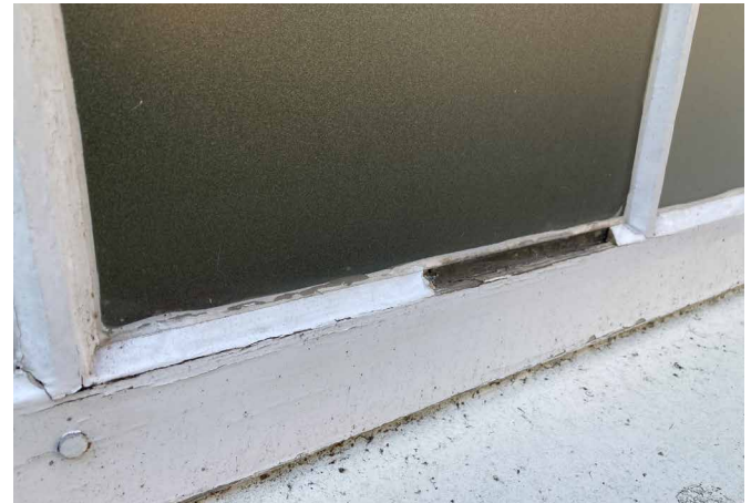
FIG. 5.18 Putty in wooden windowframe (in need of repair) / Photo: W. J. Quist
