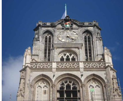
FIG. 2.13 The lantern of the Laurens Church tower in Rotterdam after conservation / Photo: W. Quist
