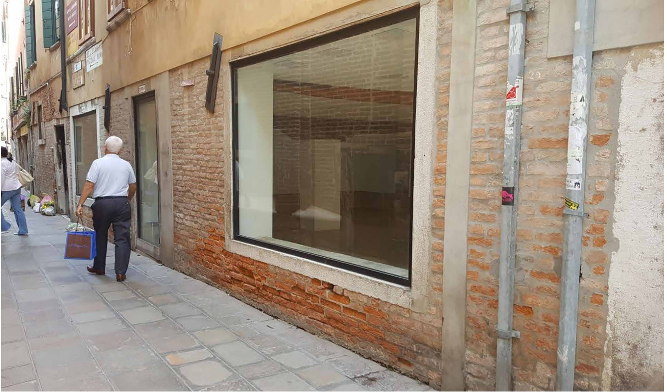
FIG. 3.1 Salt crystallization damage due to the presence of salts and rising damp, Venice, Italy / Photo: B. Lubelli
