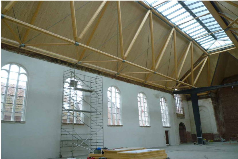
FIG. 3.12 Interior of the Elleboog church: water used to extinguish a fire had accumulated on the concrete floor and risen up in the wall, leading to a moisture content distribution similar to that observed in the presence of rising damp from groundwater / Photo: B. Lubelli
