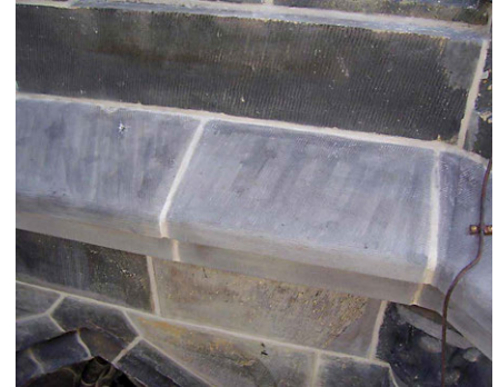
FIG. 2.14 Artificially patinated Bentheim sandstone on the lantern of the Laurens Church tower in Rotterdam / Photo: T.G. Nijland
