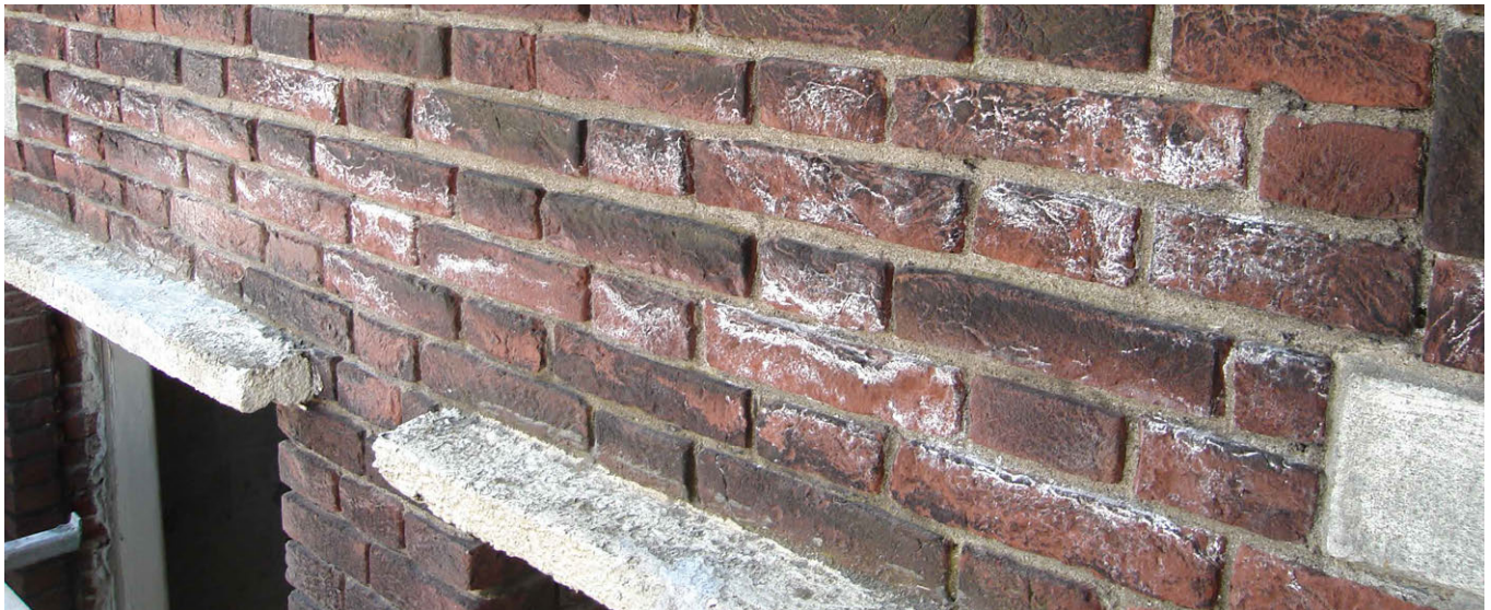
FIG. 4.28 Salt efflorescence, evidence of the presence of salts in the masonry, further confirmed by chemical analyses / Photo: B. Lubelli
