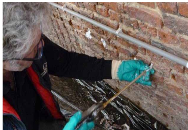
FIG. 3.6 Injection of a liquid product by means of impregnation with a product in the form of a cream / Photo: B. Lubelli
