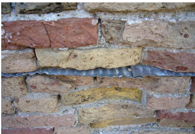
FIG. 3.4 Mechanical interruption of the wall by the use of undulated steel sheets, Venice, Italy / Photo: R. van Hees
