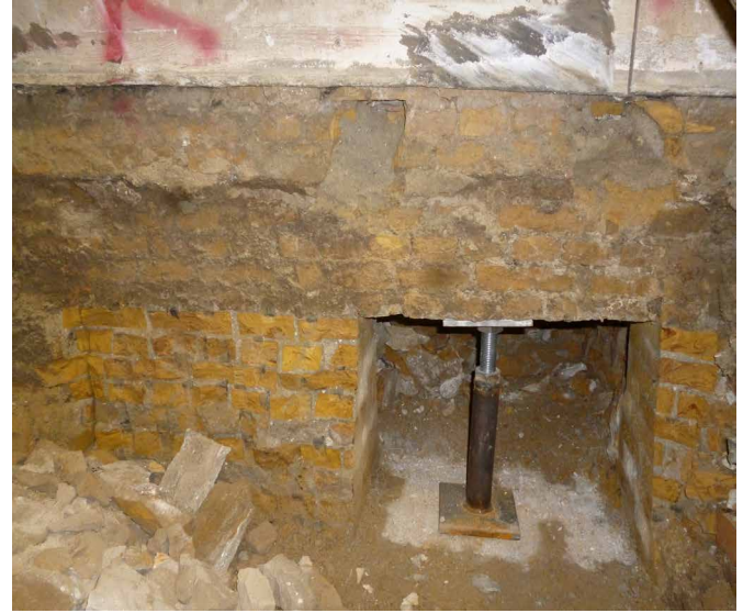
FIG. 3.11 Huis Nolet, basement: temporary support of the wall during insertion of concrete floor (December 2016) / Photo: B. L.ubelli
