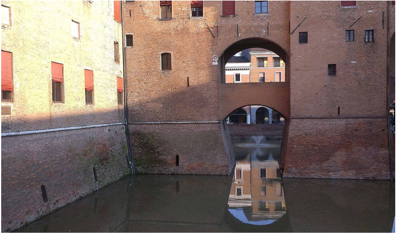
FIG. 3.2 The height of rising damp is generally limited to 1,5-2 meters, Ferrara, Italy / Photo: B. Lubelli
