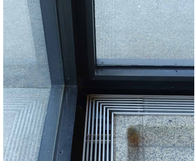
FIG. 5.40 New National Gallery, Berlin: New facade with a single glazing in a thermally non-separated construction / Photo: F. May
