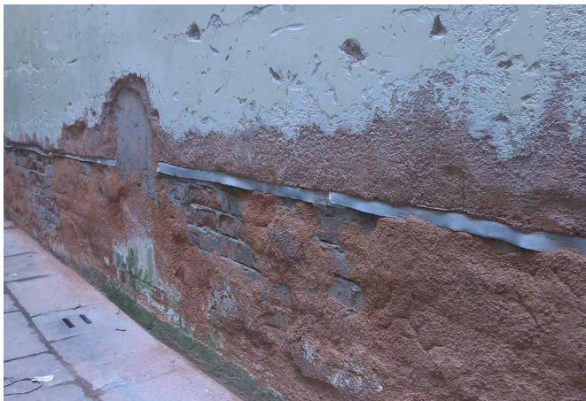
FIG. 3.3 Mechanical interruption of the wall by the use of plastic sheet, Venice, Italy / Photo: B. Lubelli
