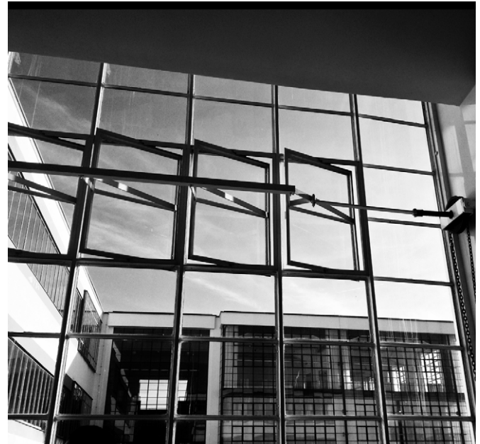
FIG. 5.8 Bauhaus Dessau, staircase, office and workshop glazings were originally using polished plate glass to achieve a precise and industrial look / Photo: pixy.org
