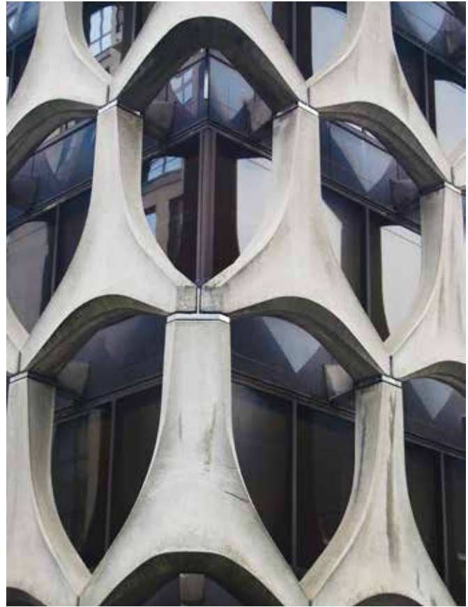
FIG. 3.28 The curtain wall composed of prefabricated wishbone-shaped elements (Ergon) of the former ALSK Bank, Brussels, designed by Marcel Lambrichs / Marieke Kuipers
