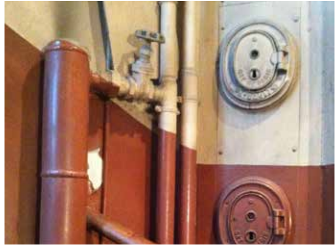
FIG. 3.42 Services in the servants' stairway of a multi-storied 19 th century apartment building, Paris / Marieke Kuipers
