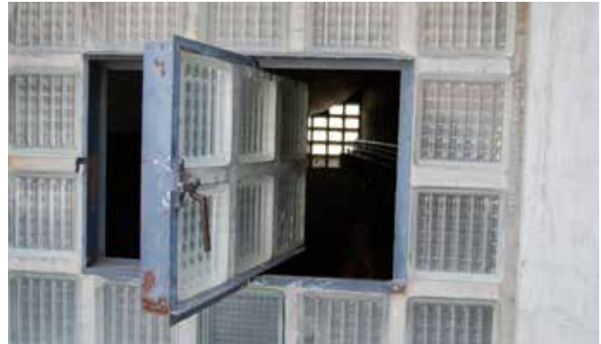
FIG. 4.10 A typical detail of modern heritage: a steel framed window with traces of corrosion in a wall of glass bricks, part of the Salime Hydro Power Plant / Marieke Kuipers
