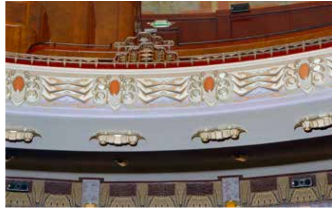
FIG. 4.13 The restored cinema hall of the Art Deco Tuschinski theatre at Amsterdam (originally built in 1921), with murals by Pieter den Besten (recently restored) and new emergency exit light / photo: courtesy of the Cultural Heritage Agency of the Netherlands
