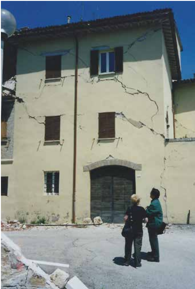
FIG. 3.1 Typical earthquake damage pattern: diagonal cracks in two different directions and X shaped cracks (house, Umbria, Italy) / photo: R. v. Hees
