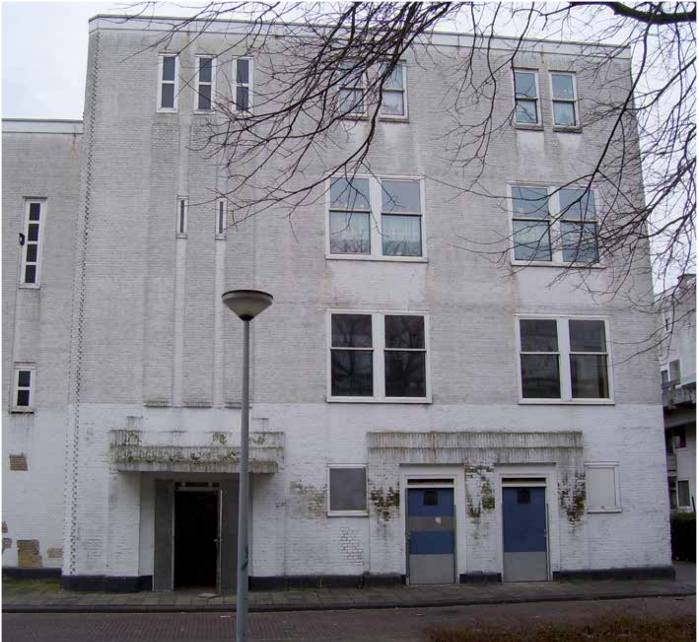
FIG. 6.15 Façade of one building showing damage (2009); to the left: paint removal - try out (Justus van Effen complex, Rotterdam, The Netherlands) / photo: A. Acquebord
