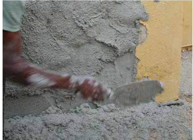
FIG. 4.14 Application of new render (house at Charloo, Curaçao, Caribbean) / photo: R. v. Hees
