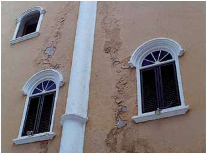
FIG. 4.7 Damage to the plaster (synagogue, Curaçao, Caribbean) / photo: R. v. Hees
