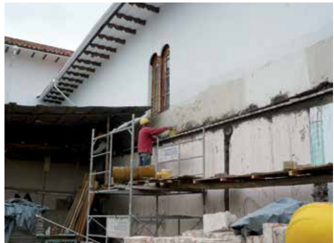
FIG. 2.12 Use of adobe for renders in a recent restoration (2010) (building in Cuenca, Ecuador) / photo: R.v. Hees
