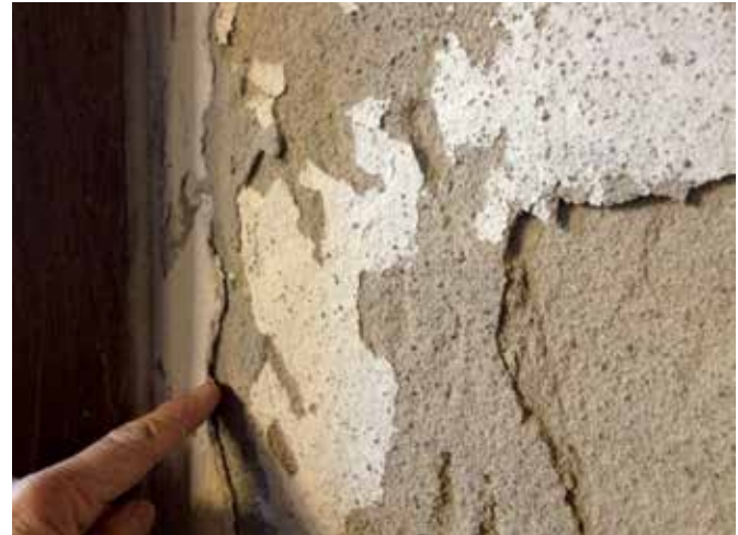
FIG. 7.5 Loss of adhesion and crumbling of plaster applied on a salt loaded substrate / photo: R. v. Hees
