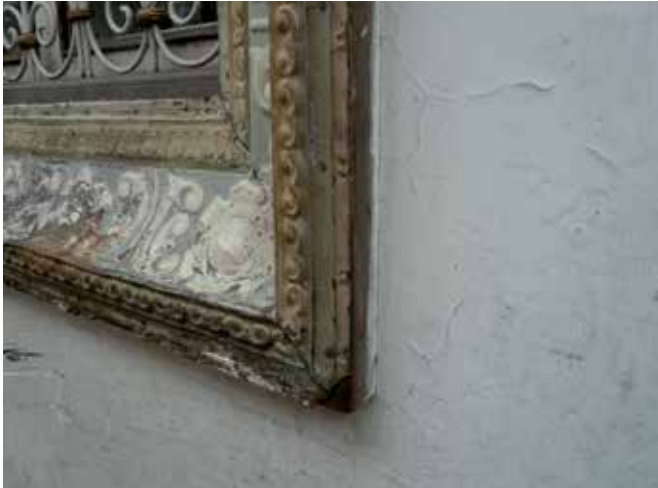
FIG. 2.7 Detail of window frame (casa Palomas, Cuenca, Ecuador) / photo: R. v. Hees
