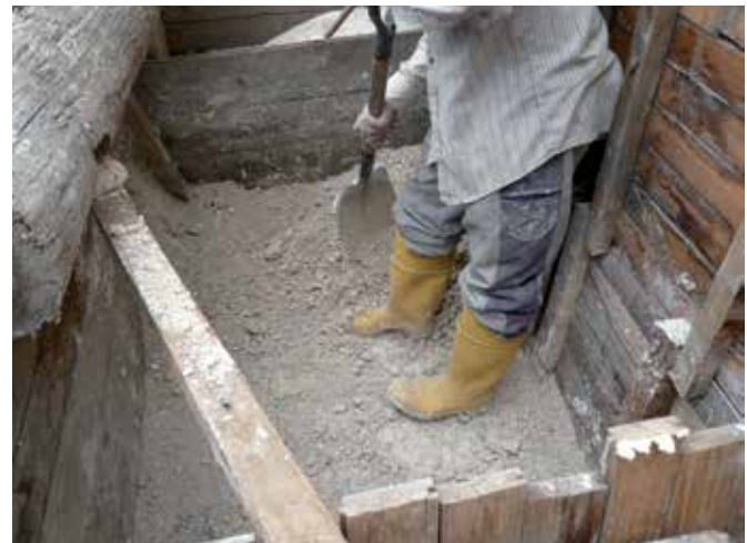
FIG. 2.14 Production of adobe for renders in a recent restoration (2010) (building in Cuenca, Ecuador) / photo: R.v.Hees
