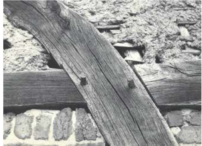
FIG. 2.21 Wattle and daub on a wooden lattice (house, south of Limburg, The Netherlands) / photo: R. v. Hees
