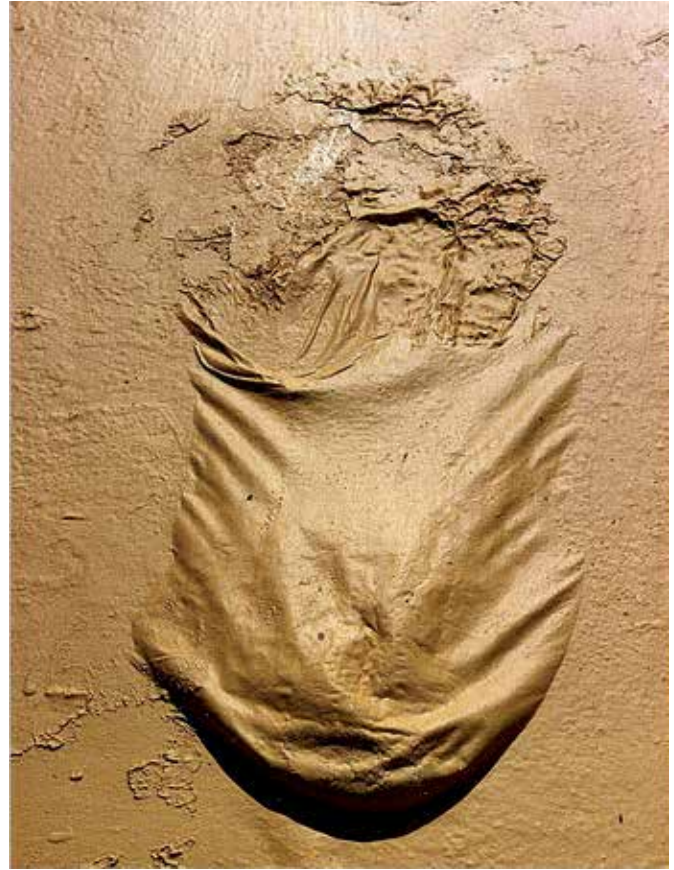
FIG. 4.6 Blistering of latex paint (detail of a painted plaster, house, Curaçao, Caribbean) / photo: R.v.Hees
