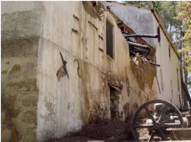
FIG. 2.16 Lack of maintenance (dwelling, Genadendal, South Africa) / photo: L.Verhoef
