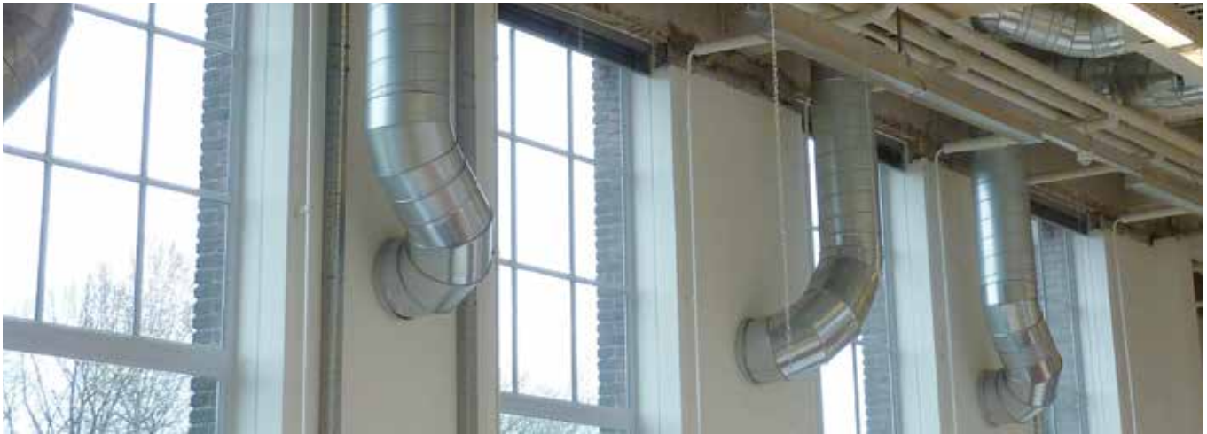
FIG. 6.27 Ventilation ducts connected with the 'lion heads' (Faculty of Architecture, TU Delft, The Netherlands) / photo: S. Jansen
