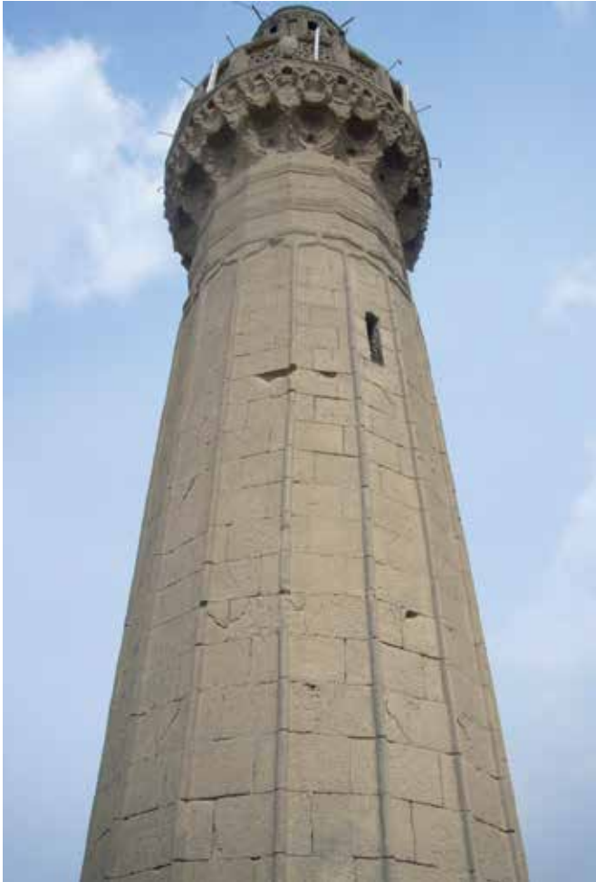
FIG. 3.5 Diagonal cracks in different directions, visible after the 1992 earthquake (minaret, Al Faqahani mosque, Cairo, Egypt) / photo: R. v. Hees
