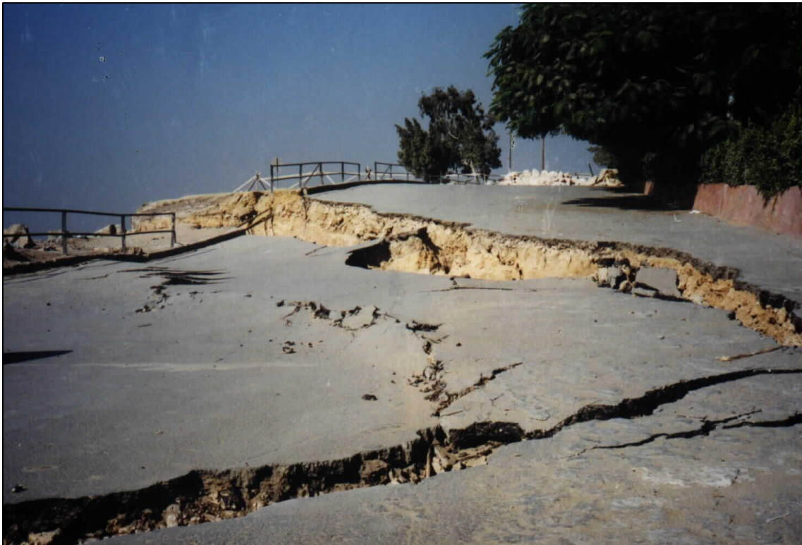
Figure 2-4: Soil failure (www.4isfge.org).
