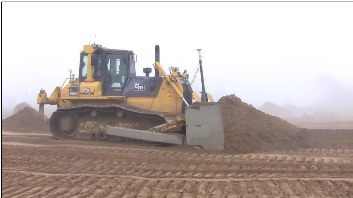
Figure 2-56: An example of passive soil failure, the Komatsu D65PX-15 ( www.youtube.com ).
