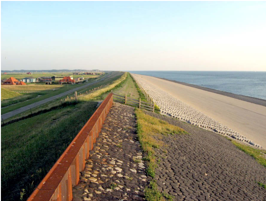
Figure 10.30: Additional sheet piling at crest of dike, Hondsbossche and Pettemer sea defence. From Wikipedia, uploaded in 2005 ('Credits' on page 575).
