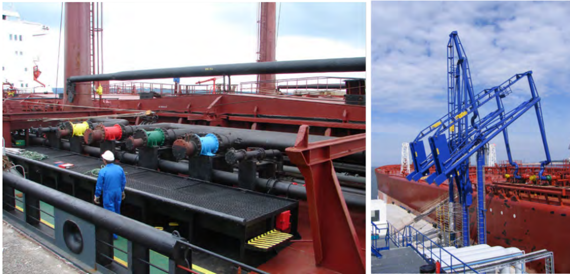
Figure 5.3: Liquid bulk (un)loading facilities; left: manifold ( Maya OBO carrier 3 by Herv Cozanet is licenced under CC BY-SA 3.0); right: (un)loading arms ( Marine Loading Arm KLEa by Ljl.kanon is licenced under CC BY-SA 3.0).
