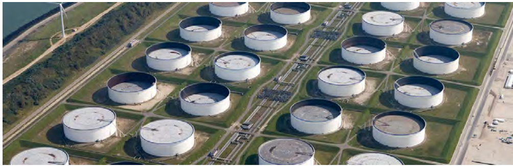
Figure 5.6: Containment bunds around oil storage tanks at the Maasvlakte Oil Terminal in the Port of Rotterdam (from www.vopak.com , Maasvlakte Olie Terminal (Rotterdam) by Vopak. Copyrights 2021 Royal Vopak.).
