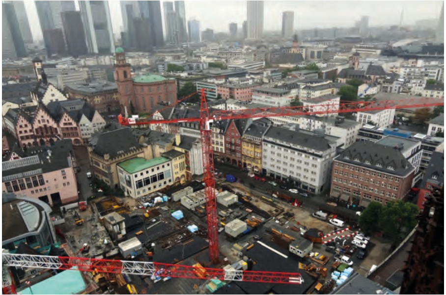
“Old town” construction site photographed from the cathedral, 2014 photo credit: Monika Motylinska
