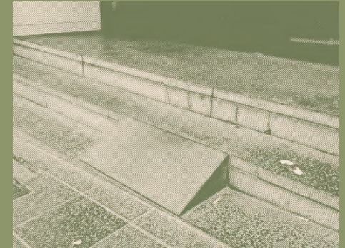
INACCESSIBLE WHEELCHAIR RAMP - PLACE LIEDTS - BRUSSELS PHOTO BY AUTHORS
